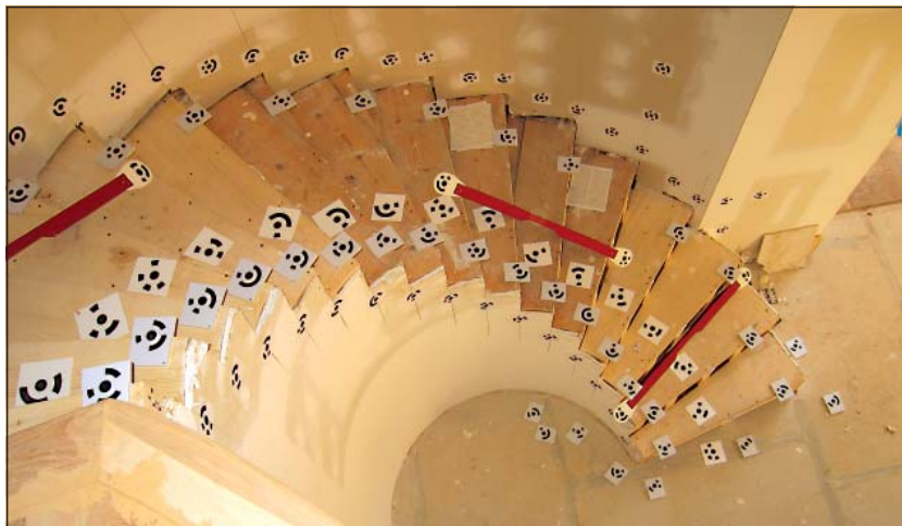
A perfect curve — Chris Morley of Royal Oak Stairs uses the ETemplate system for accurately measuring curved stairwells so he can create the various stair components.
